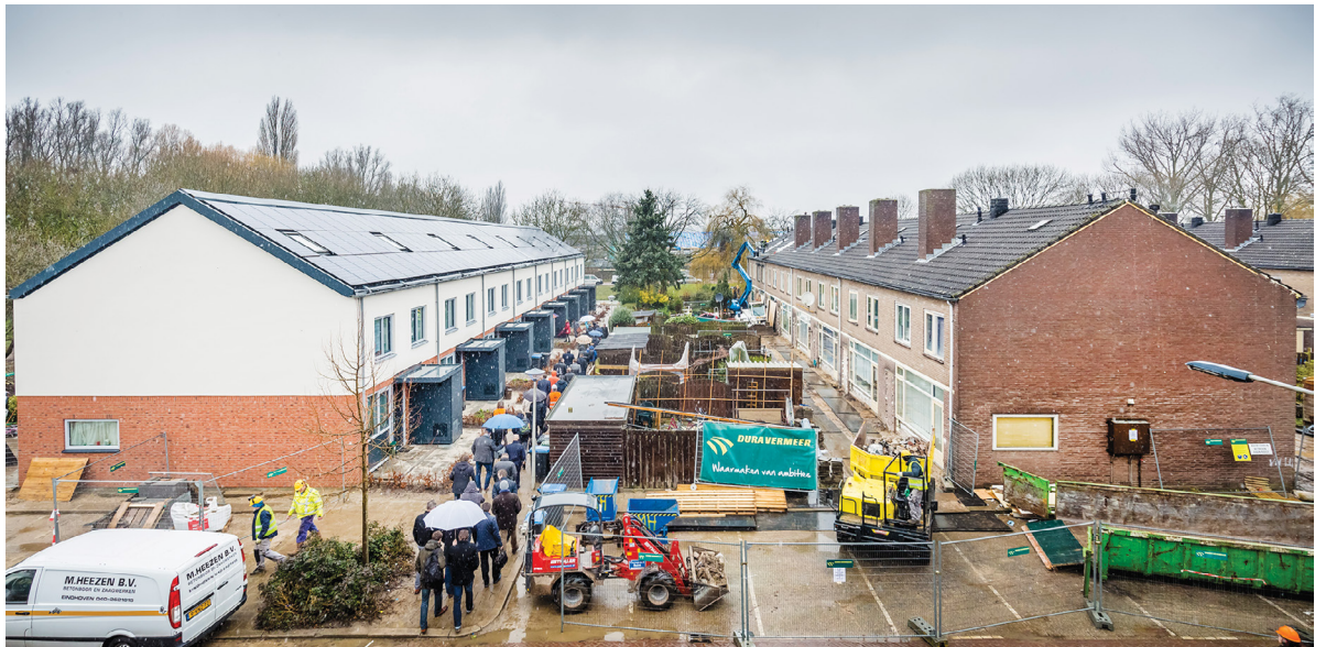
A row of Energiesprong retrofits (left) in the Netherlands (image courtesy of Energiesprong)
